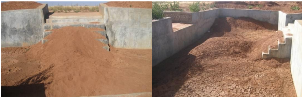
Plate 2. Siltation of Haffir dam in Lankerta
