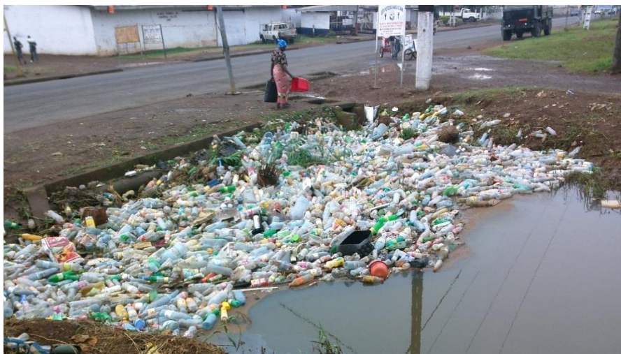
Figure 5. Urban culvert along Manga William Street, Limbe. The constricted nature of the culvert dimension stands at the origin of river blockage. Only culvert enlargement can ensure the free passage of water downstream
