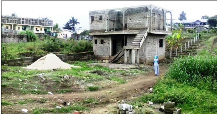
Figure 4. Buildings Construction astride the dry valley Interfluves near Blessed Hostel along Chief Street, Bomaka. The House is protected by a short concrete wall near the base to prevent an inundation of the lower portion of the house
