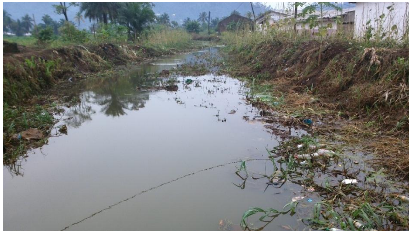
Figure 1. Flow channel of the Jengelle Stream through the Limbe New Market. The narrow and shallow channel along Manga William Street accounts for the repeated and rapid over-floods during the rainy season
