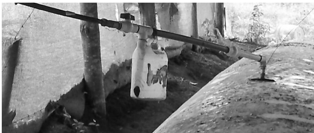
Figure 2. Gas Pressure Relief Valve for Biodigestion System A
