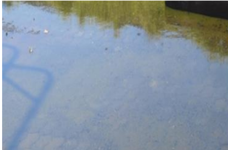
Figure 2. The standing water forming swampy conditions
