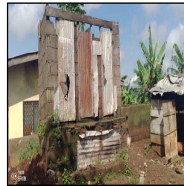
(iii) Poorly constructed
