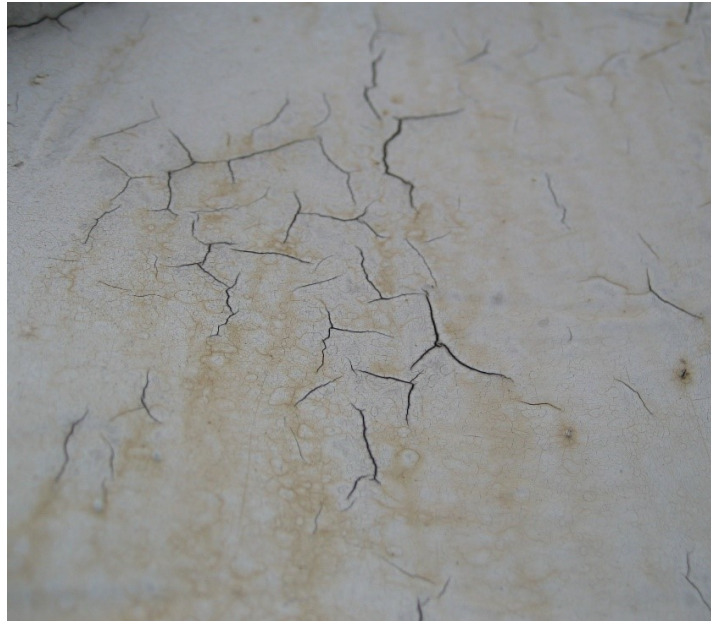
Figure 6. Cracks and creases in paint due to age and wear (slightly modified). Dynamic deformation of the underlying surface would exacerbate these features.
