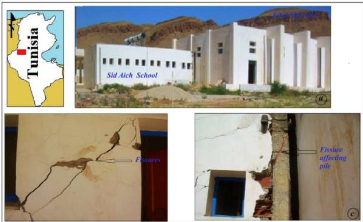
Figure 2. (a) location of Sidi Aich school; (b) Fissures affecting the walls of the school ; (c) Fissure affecting the piles of the school
