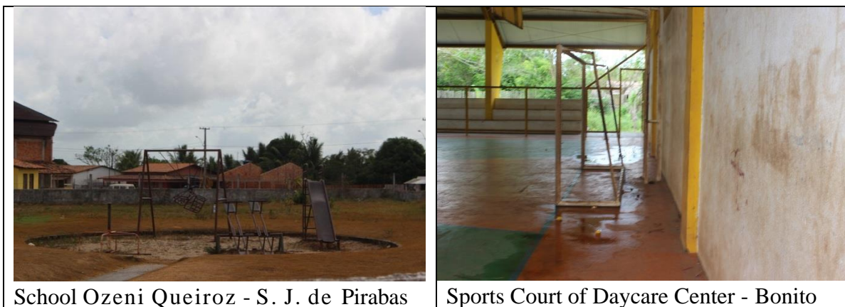
Figure 5. Examples of completed, however, deteriorated buildings in November/December 2017.
