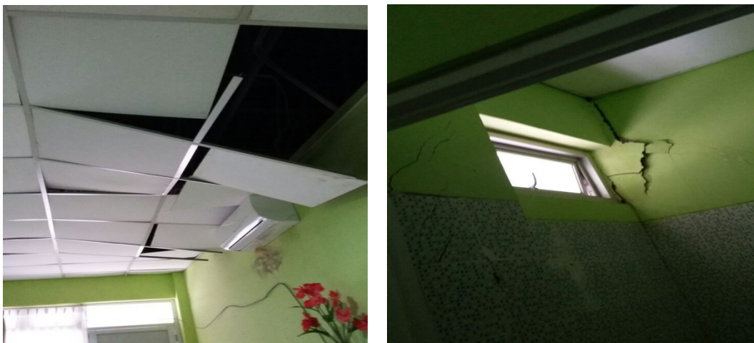
Figure 4. Damage to most space Muko-Muko Regency RSU earthquake June 2, 2016. (Archives of MDMC Bengkulu, June 2, 2016)
