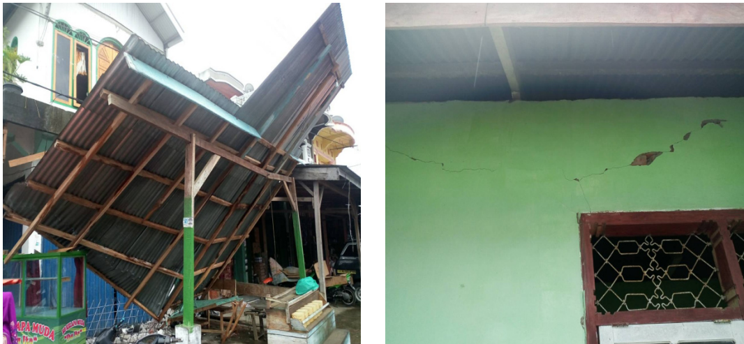
Figure 3. Most houses in Muko-Muko Regency damaged by the earthquake of June 2, 2016 (source: Documentation Archives of MDMC Bengkulu)
